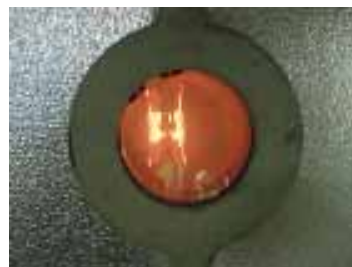
Boiler viewing window
