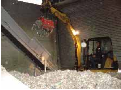
Recovered paper rejects fed to fuel preparation plant
